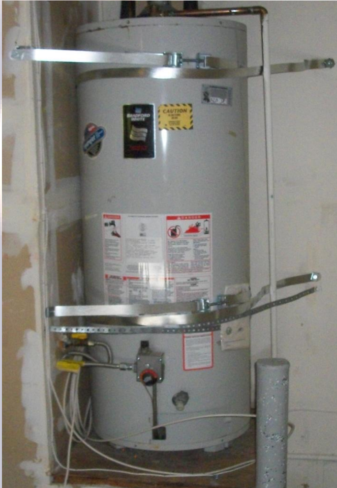
Tank Water Heater
